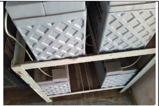
Batteries stacked without ventilation.
