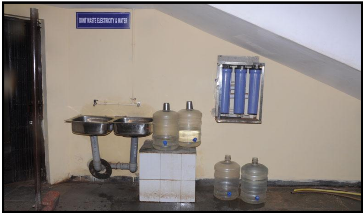
RO WATER PLANT IN LADIES HOSTEL
