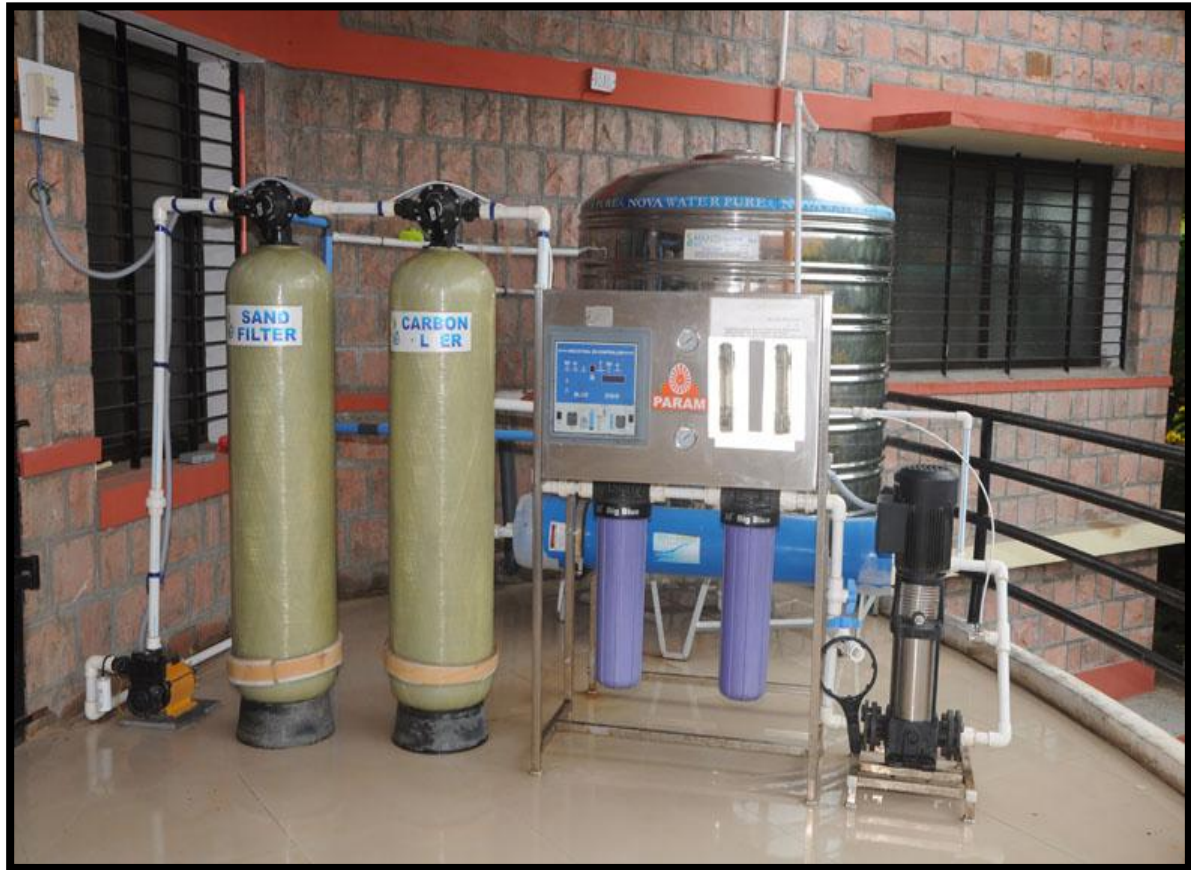
RO WATER PLANT WITH CAPACITY 2000 ltrs in
