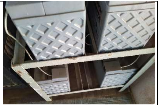
Batteries stacked without ventilation.
