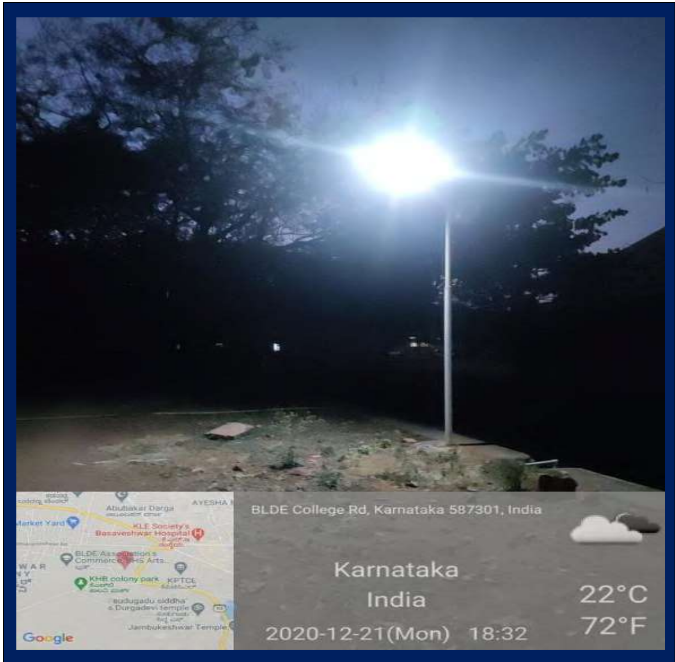
PICTURE 2 : SENSOR BASED STREET LIGHTS RIGHT SIDE OF SWIMMING POOL
