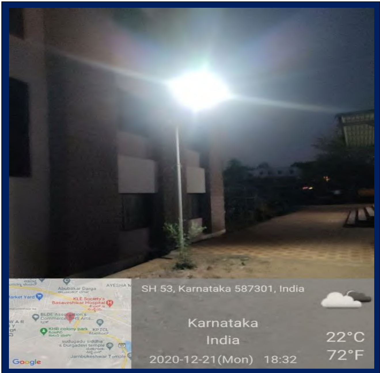
PICTURE 1 : SENSOR BASED STREET LIGHTS RIGHT SIDE OF SWIMMING POOL
