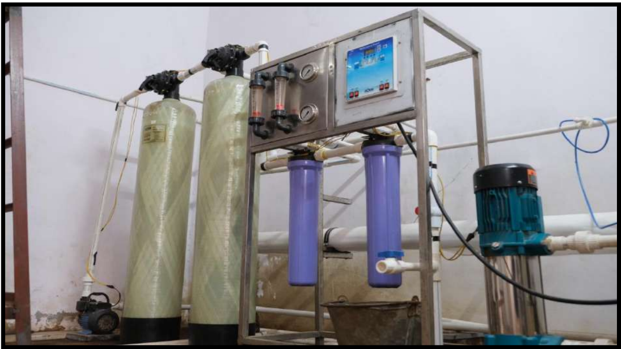
PURIFIED R O WATER PLANT IN COLLEGE CAMPUS WITH 4000 LTRS CAPACITY IN CAMPUS
