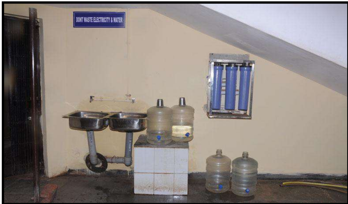
R O WATER PLANT IN LADIES HOSTEL
