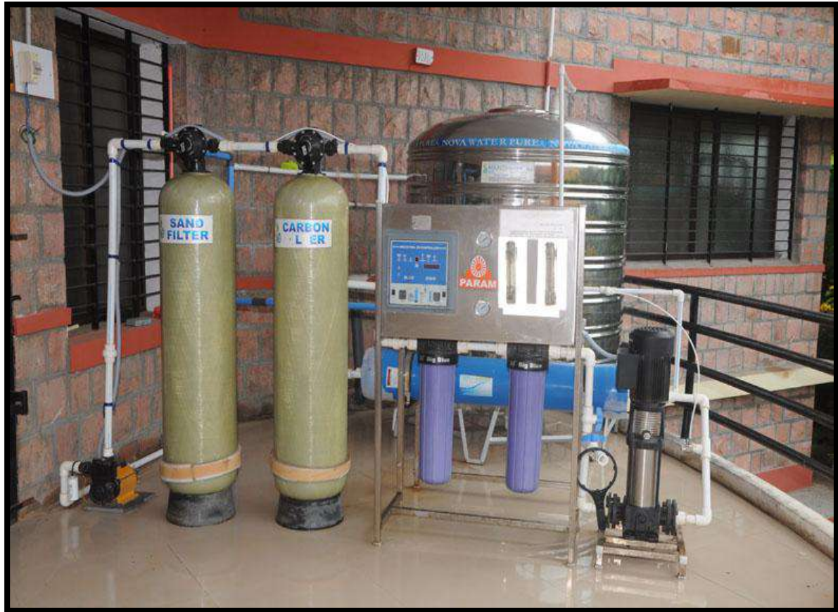
R O WATER PLANT WITH CAPACITY 2000 ltrs in
