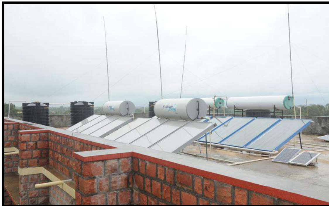
SOLAR HOT WATER PANEL WITH 10 UNITS , EACH ONE HAS 100 LTRS CAPACITY
